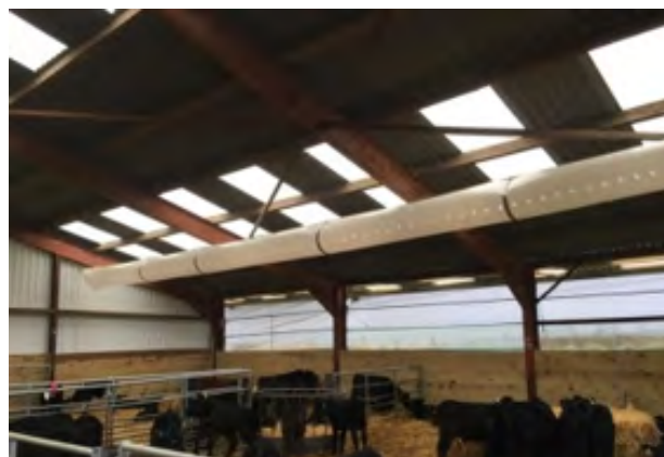
Figure 15: Example of a PPTV system in operation
