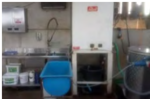
Figure 23: Example of a well designed equipment cleaning area
