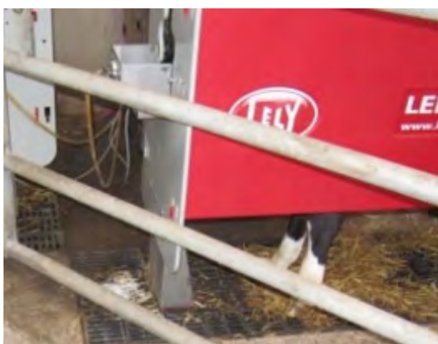
Figure 26: Automatic feeders should have well designed pipework to direct cleaning water away to drains quickly
