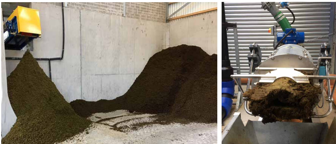
Fig 2. On farm slurry dewatering for solids export
